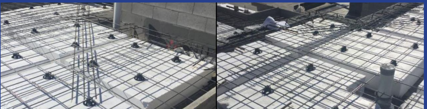
Projects: Coomera Urban Village Services: Geotechnical, Residential and Site Inspections Client: Ingenious Homes
